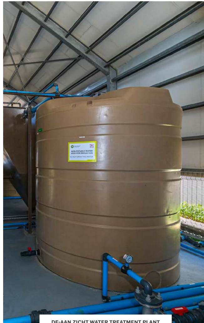
DE-AAN ZICHT WATER TREATMENT PLANT
